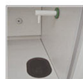
Water Tap & Water Sink
